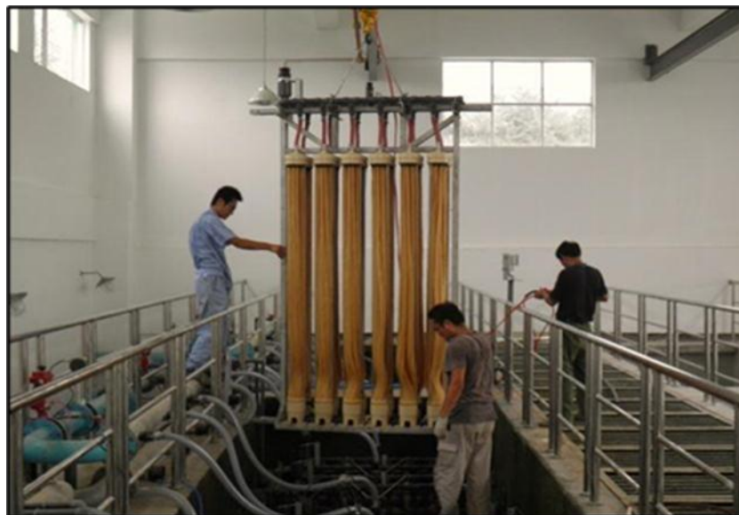
Figure-1 : Installation of the hollow fiber membrane in MBR wastewater treatment plant.
